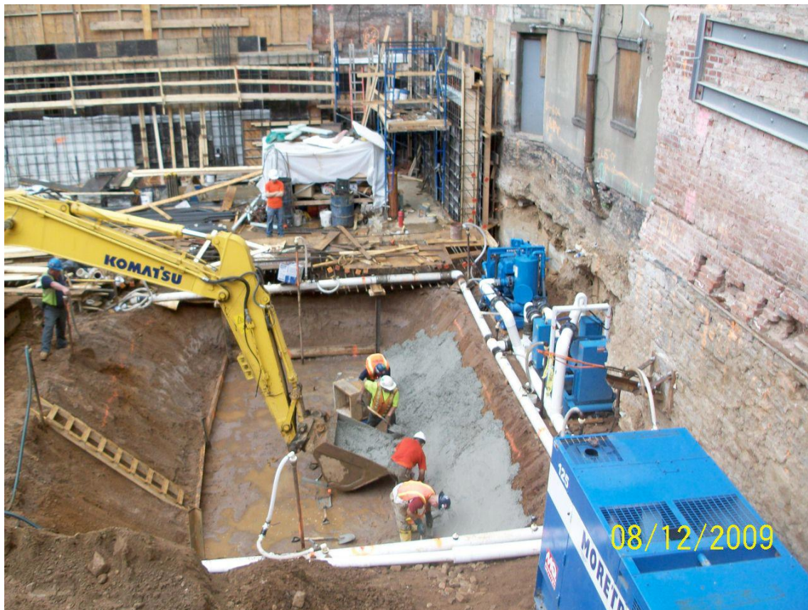
Figure 15: Display the Dewatering System
