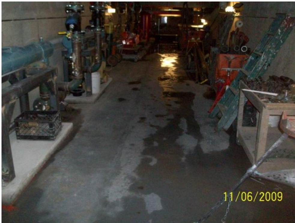
Figure 10: Illustrates the Heat Exchanger in the Neighboring Building Possessed by the Owner
