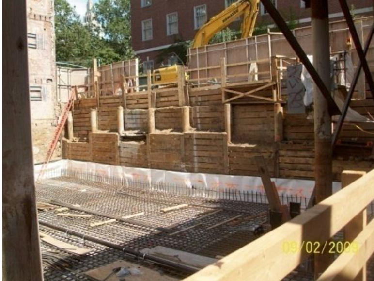
Figure 8: Shows the Sheeting (Lagging) and Piles on the East Side (Mac Dougal Street)
